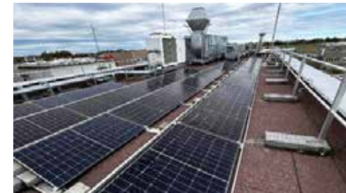
The new PV system at the new production building in Ulm.
